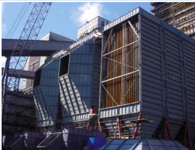
Tuzla Power Plant, Bosnia and Herzegovina. 3 boilers OB-650, units 200 MW
