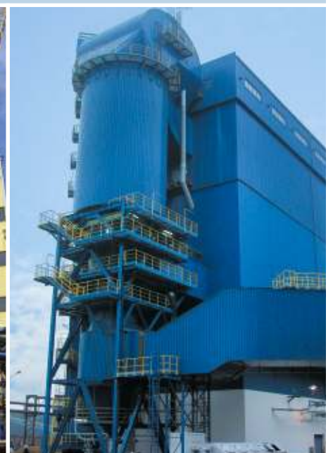
Łódź 4 CHP Plant. FGD Plant based on semi-dry method
