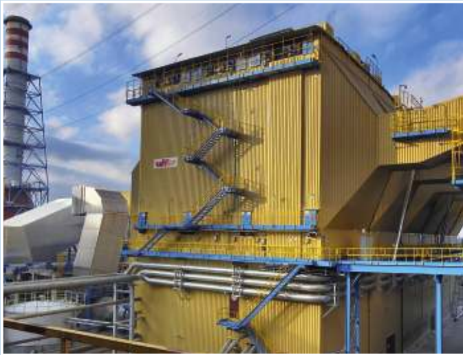
PP Kozenice - ESP of Unit no. 10 - 560 MW
