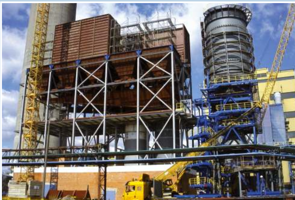
Łódź 4 CHP Plant. Bag filter erection at FGD Plant based on semi-dry method
