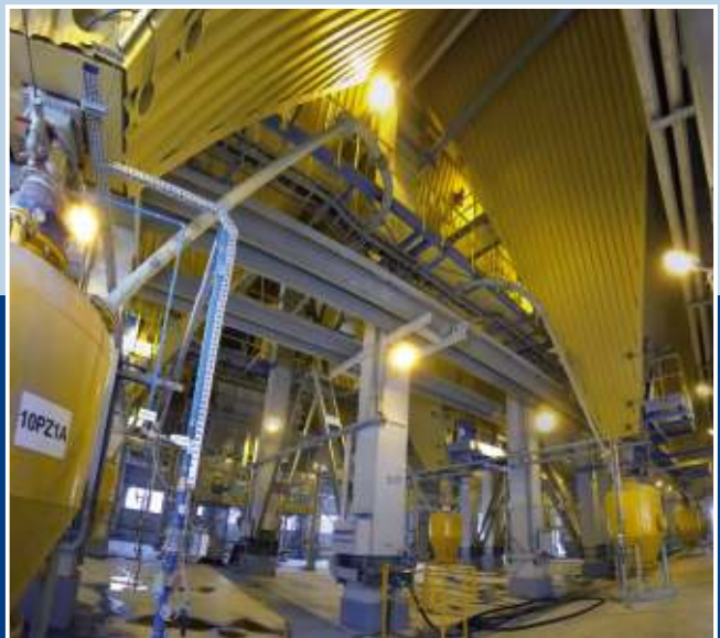
Pneumatical ash handling system in Power Plant Kozenice Unit no 10
